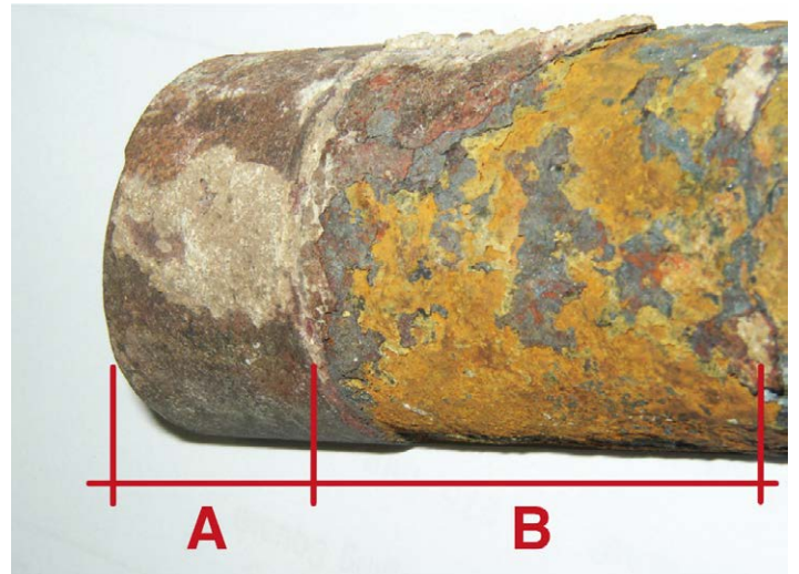
Superheater tubes from a waste incinerator.
