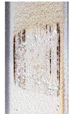
Slight coating rupture mixed with cutting and some blade material transfer
