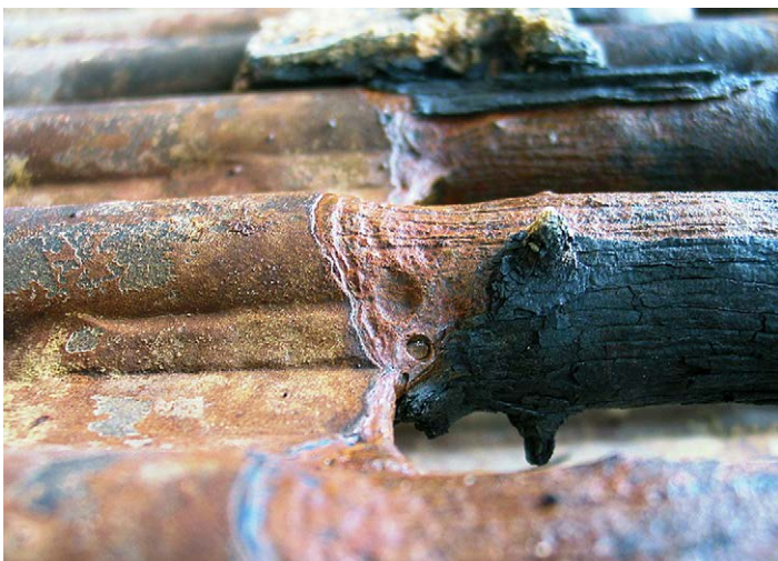
A severely corroded waterwall tubes operated without surface protection.
