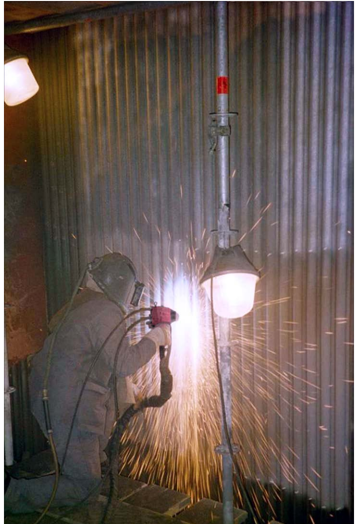
On site, manual electric arc wire spraying of a coal-fired boiler waterwall.
