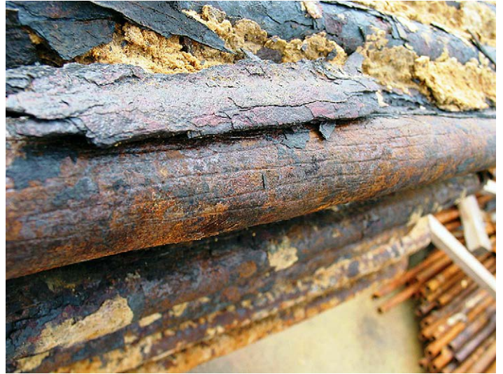
Boiler tubes that have failed as the result of severe corrosion. Note the "elephant hide" appearance of the middle tube that may be the result of fireside corrosion fatigue.
